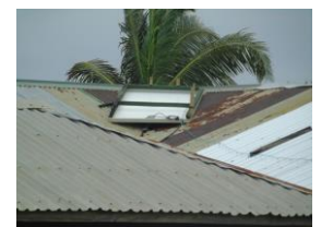
Dachpanel Comedor defekt
